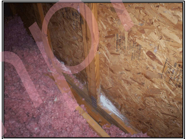
Miscellaneous photo of mold growing at other areas at the base of the right gable end siding.
