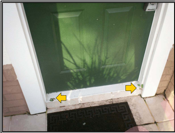
Miscellaneous photo of the live plants at the front entry near the decay damaged wood.
