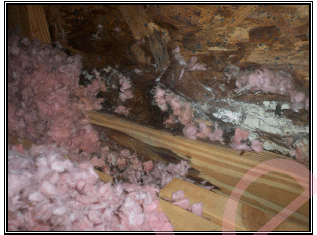
Photo 2- Another decayed section of the right gable end siding above the hall bath wall below.
