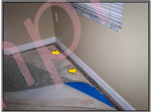
Photo 4- Decay damaged section of the moist tack strip in the right front bedroom.
