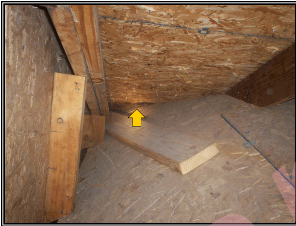
Photo 3- Wood decay at a section of roof sheathing below the base of the valley right of the garage.
