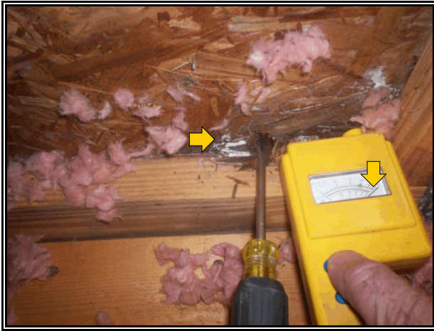
Photo 1- Wood decay and increased moisture at the base of the right gable end siding in the attic.
