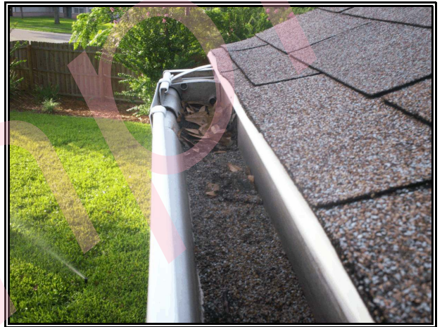
Photo 10- One of the partially clogged rain gutter runs.
