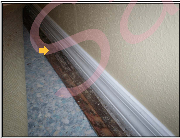
Photo 5- Decay damaged and slightly damp carpet tack strip at the front of the living room.
