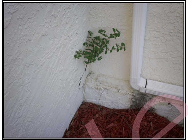
Miscellaneous photo of the plant growing in the crack at the left side of the home.
