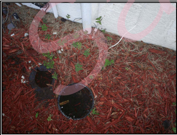
Photo 11- The missing caps at the domestic and lawn sprinkler shut off valves right of the home.
